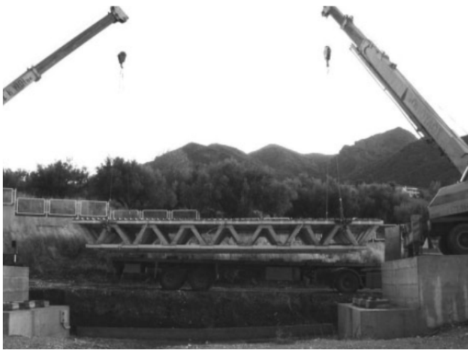
Fig. 14 – Installation of the bridge over the span with the aid of cranes. Source: [9].
